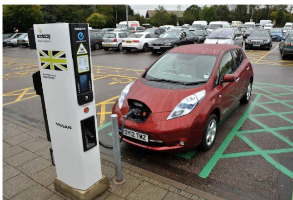
Figure 6: Electric car charging bay
